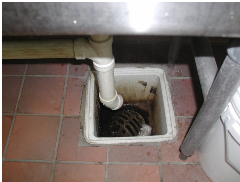
Church Annex sink floor drain
